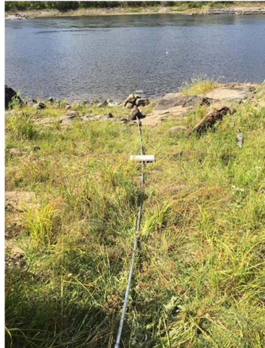
1/2 in galvanized conduit from equipment box to turbidity meter
