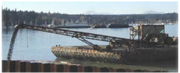
Cap material is typically put in place using equipment on a barge positioned in a river.
